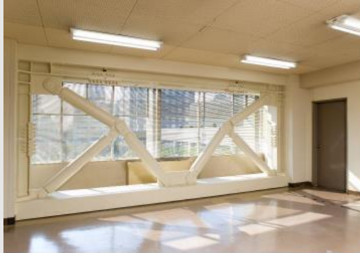
Seismic Brace with vibration damper inserted.
