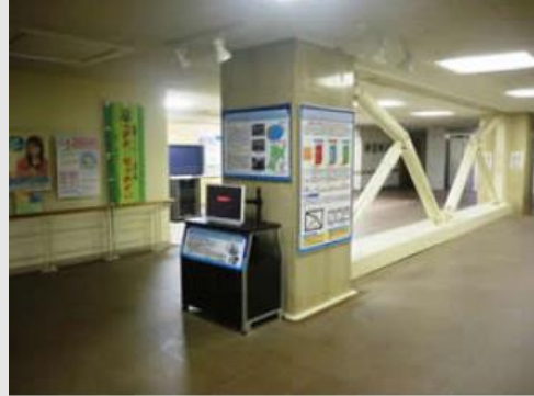
Seismic Brace & Seismometer installed on ground floor hall.
